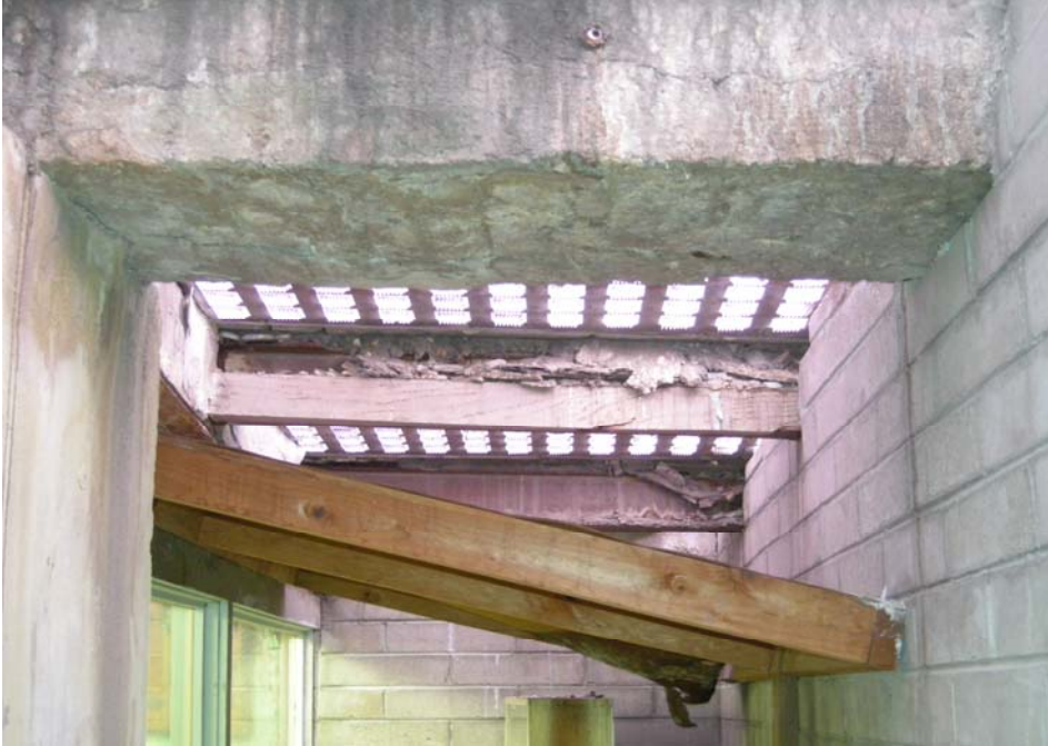
Another photo demonstrating the efforts to shore up the weakened beam supports.
