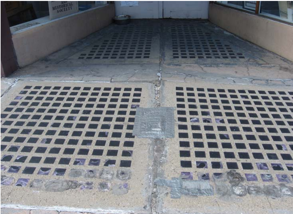
View of the entrance into the Museum. Note: Duct Tape to stop leaks into lower level.
