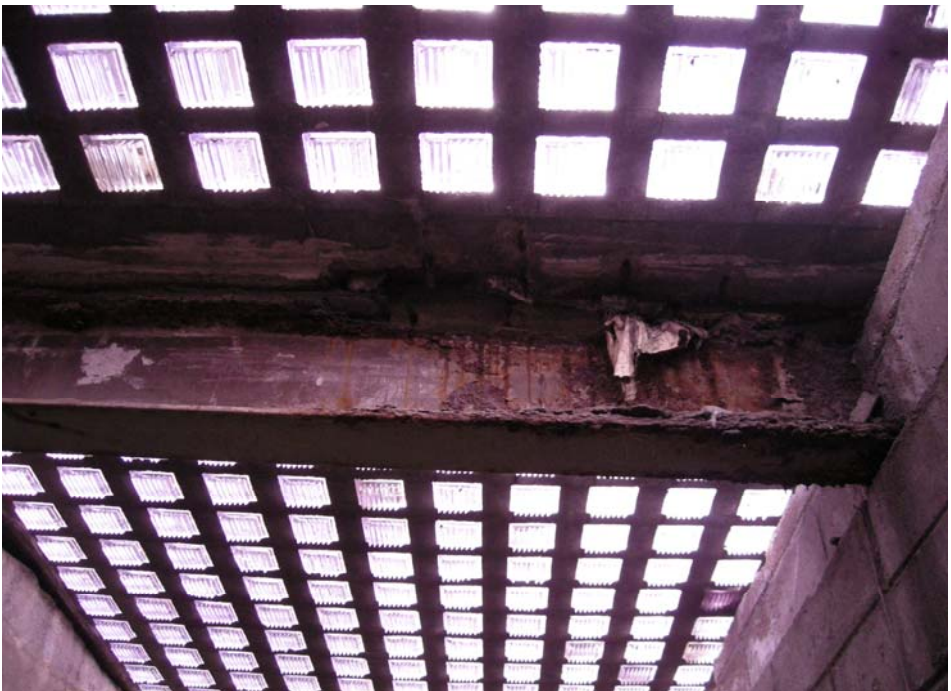
Glass Sidewalk view from basement below. Note: I-Beam corrosion.
