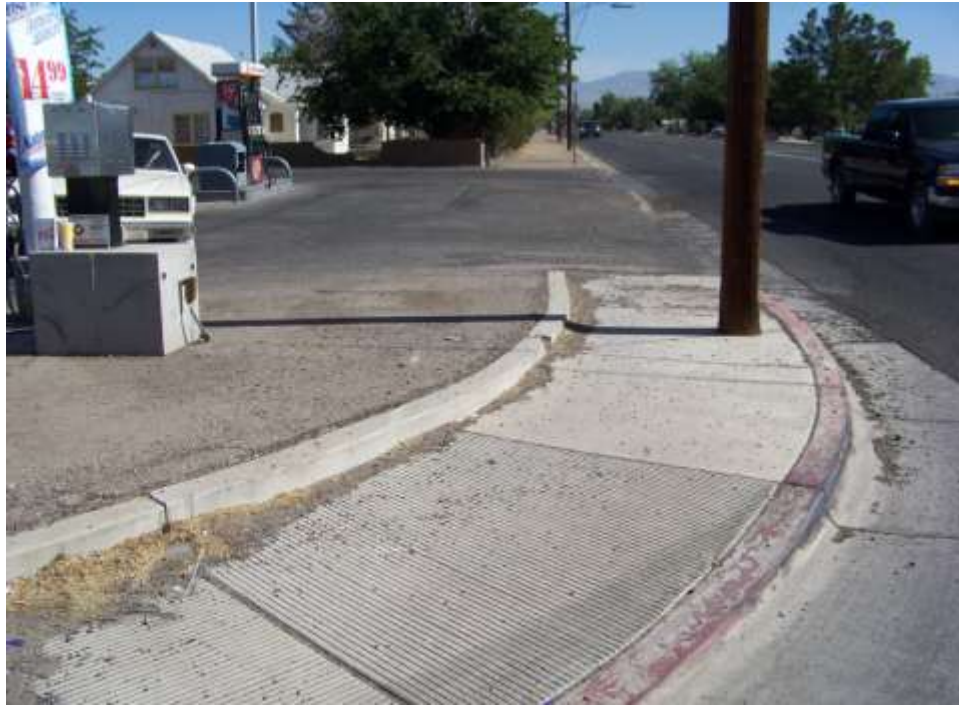
Photo #1: At Beginning of Project; Relation Street (MP 120.33) looking north in the direction of new sidewalk.
