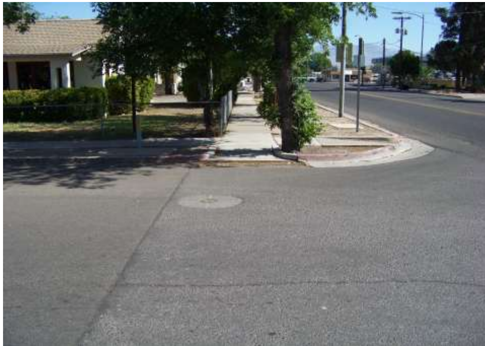
Photo #5: At Main Street looking north with US Highway 70 in the background; existing sidewalk and Sidewalk Ramps to be removed and replaced.
